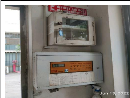
Fire Control Panel and first aid
